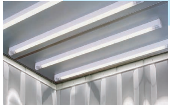
T drop fluorescent lights
